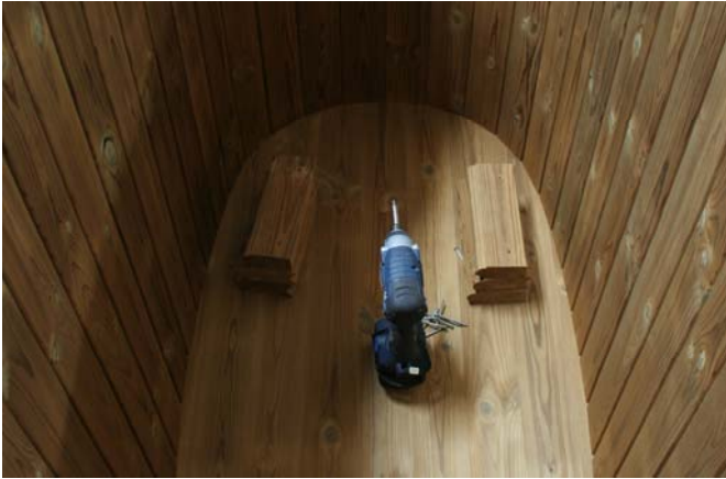
Assembly of bench. The support pieces of the seat is shown in the order they are assembled.
