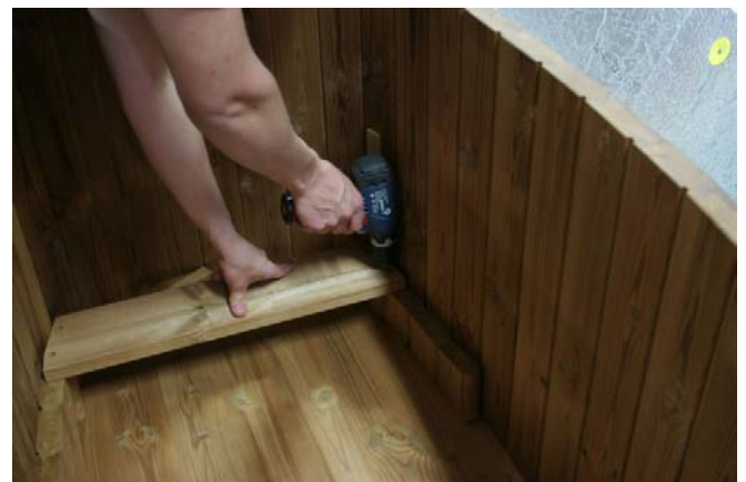
Predrill with a 3mm drill and screw the bench in place with 4 screws, don't forget to use the included washers!
