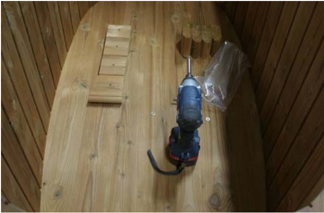
Assembly of benches. Support pieces for the bench are shown in order of assembly.
