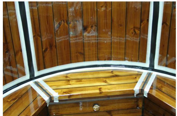
5. The sides are assembled and a joint is made with sealer around the seating well and sides.
