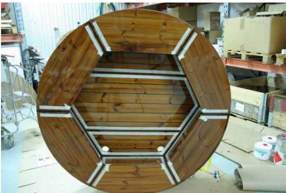
3. Mix up 50 ml Comp. A and 12.5 ml Comp. B and apply the coating over the joints. HINT! Turn the base on it's edge to see better. First hold the brush so it covers the joint and then so the coating is also applied outside the joint itself.
